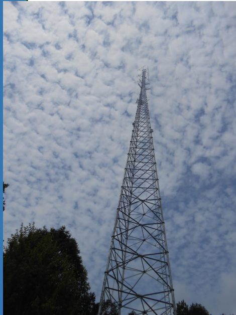
The new tower addresses radio coverage gaps and improves reception for police, fire and EMS emergency communications.
